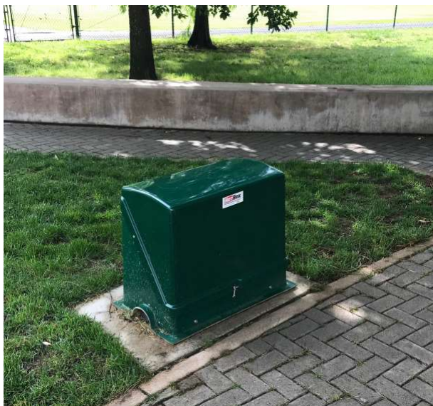
Securing cover for above grade backflow preventer
