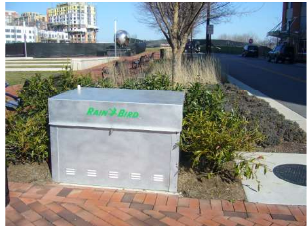
Above grade irrigation backflow preventer enclosure
