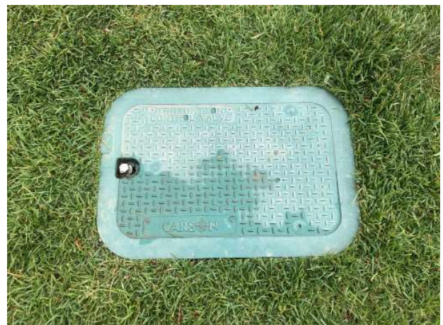
Below grade irrigation securing enclosure
